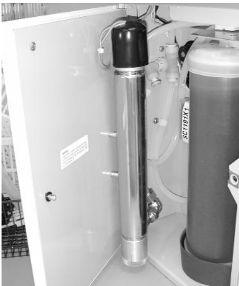
UV Lamp Installation
